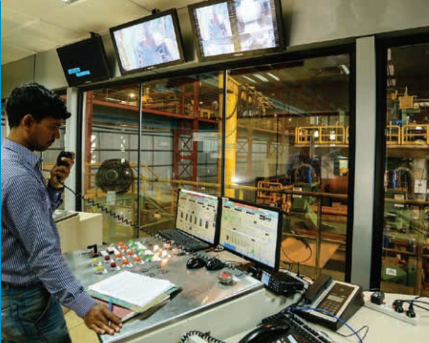
Control Room at CRM II Vijayanagar
